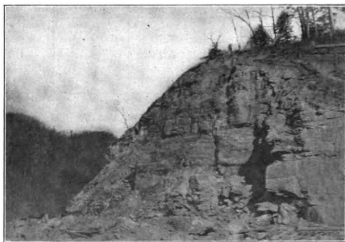
Disintegrated Rock in Elmore Cut; Deepwater Railway.
